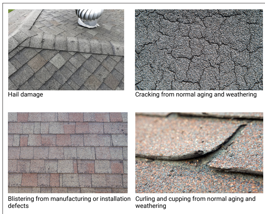
Figure 2-28 Images showing various types of shingle damage (From shutterstock.com/JLStock; iStock.com/RonTech2000; iStock.com/xphotoz; iStock.com/BanksPhotos)
